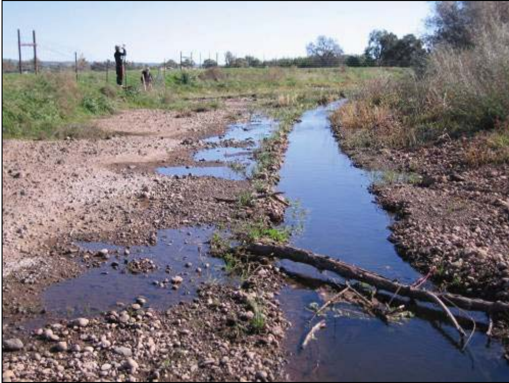
Figure C-69. Inset channel excavated within a wide and shallow plane bed reach to concentrate low flow and increase flow depths.
