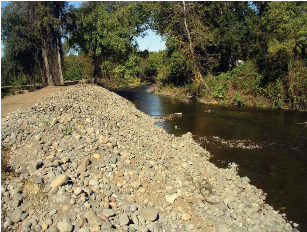
Figure C-34. Channel modified by heavy equipment excavation in Reach 1 of Craig Creek.
