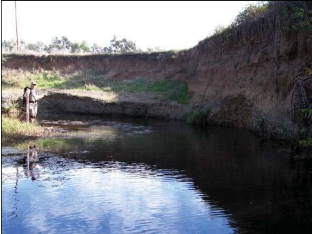
Figure C-7. Eroding bankline in Reach 4 of Antelope Creek.
