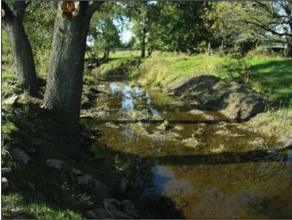
Figure C-49. Potential barrier B4. Excavation of alluvial sediment in Reach 1 of Butler Slough.
