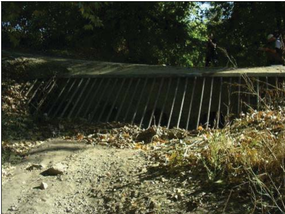
Figure C-52. Potential barrier B6. A road-stream crossing in Reach 2 of Butler Slough.
