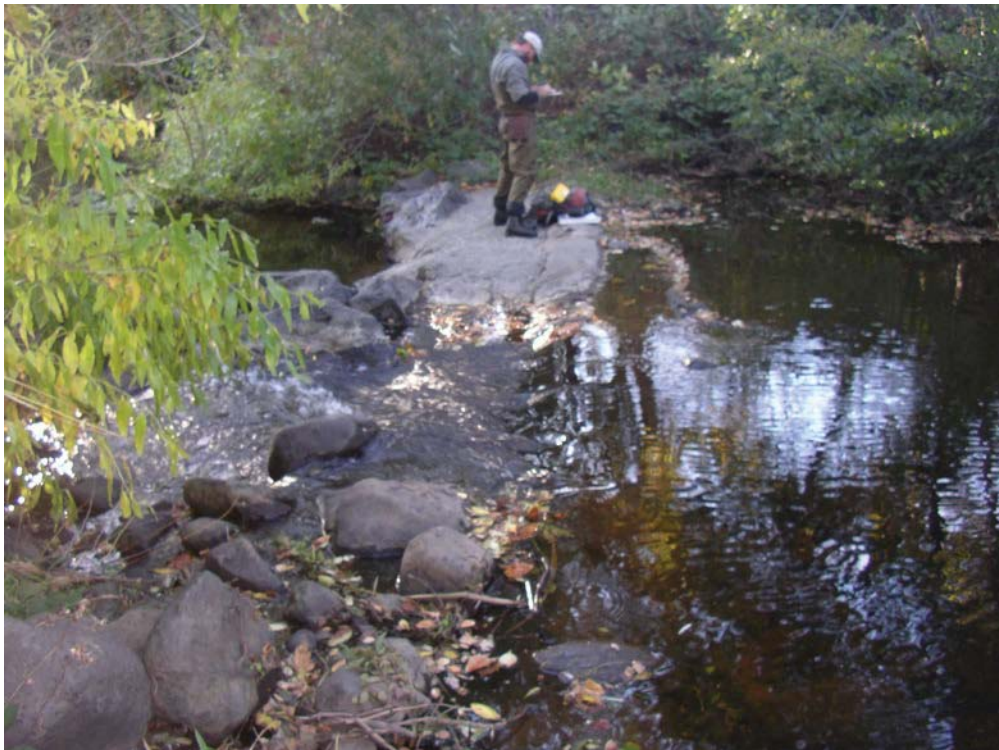
Figure C-28. Potential barrier A12 (fall 2009). Concrete apron embedded with a water pipe crossing the channel in Reach 3 of Antelope Creek upstream of Kauffman Avenue.
