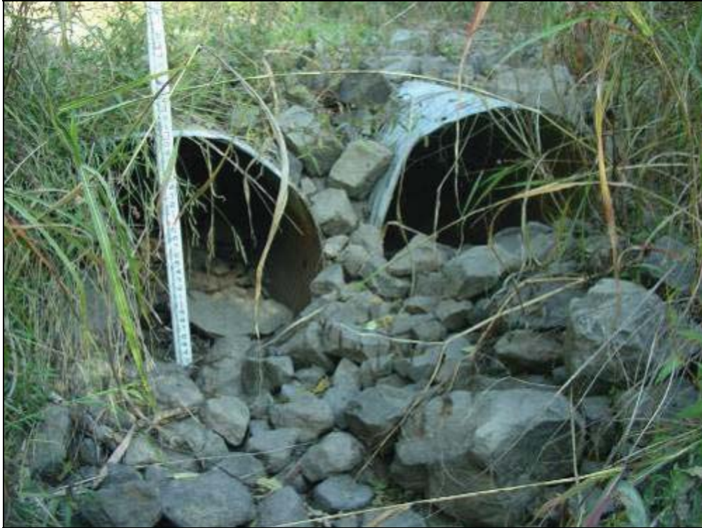
Figure C-51. Potential barrier B7. A road-stream crossing in Reach 2 of Butler Slough.
