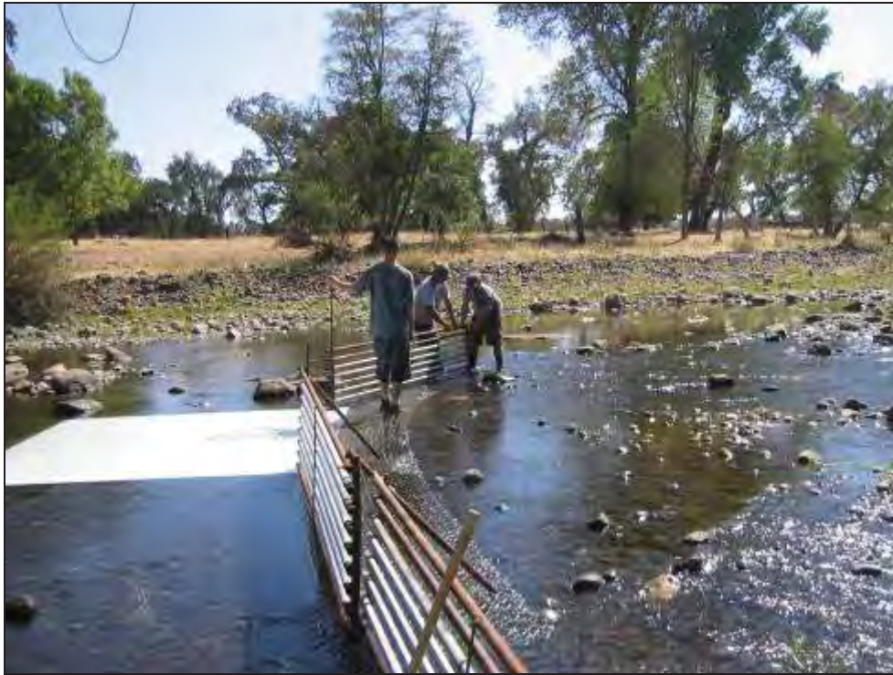
Figure 10. Construction of a weir included white high density polyethylene (HDPE) sheets staked to the creek bottom to make the observation of passing salmon easier.
