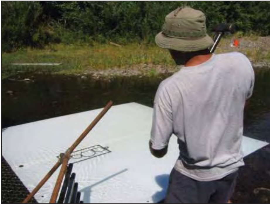
Figure 9. Construction of the weir. Dog leg fittings were bolted to the uprights and the “weir arm” slides through the fitting and was pounded into the stream bottom at a 45 degree angle downstream.
