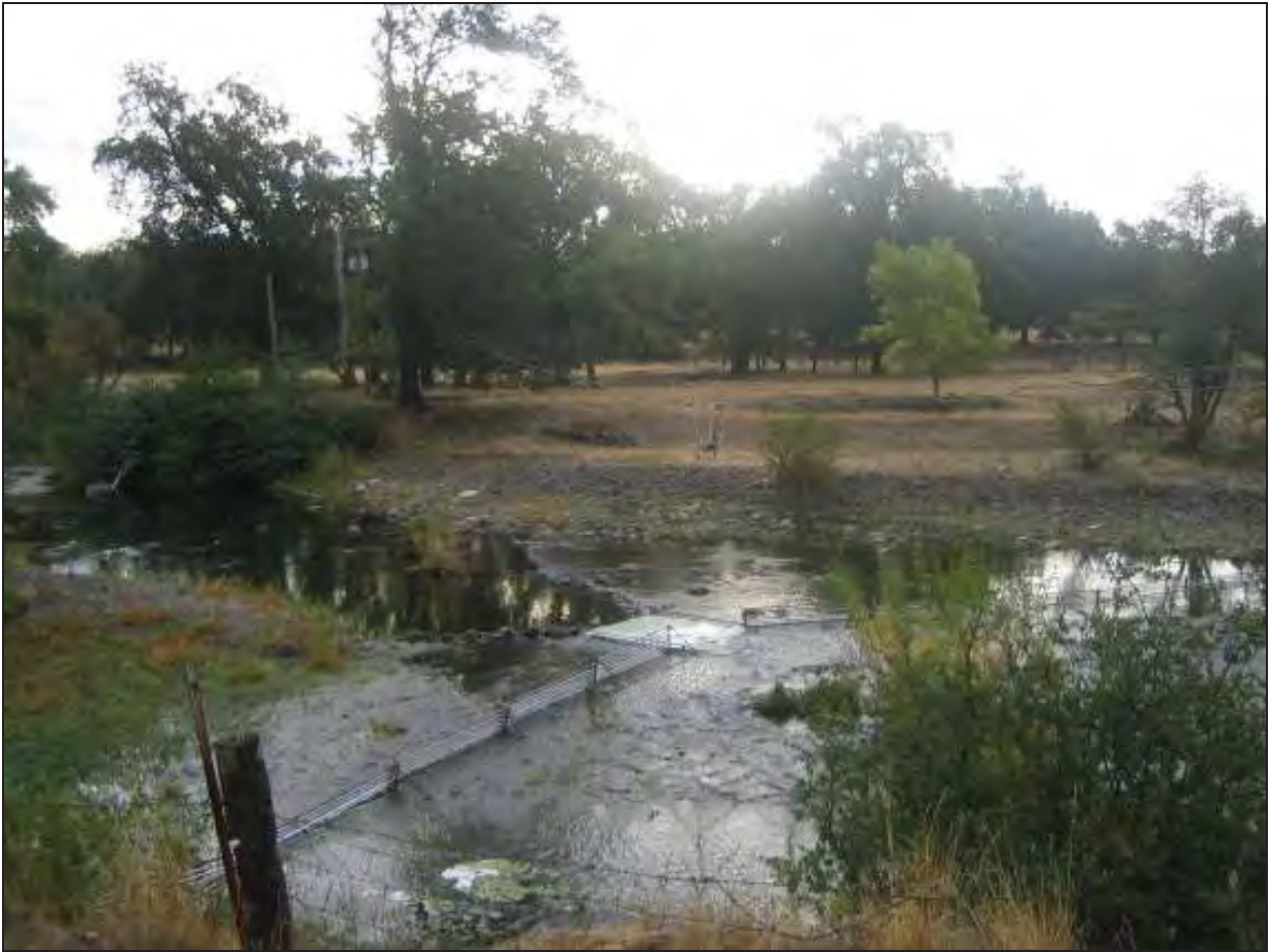
Figure 5. Bear Creek video station power supply box. Cables were used to suspend the camera directly over the weir's fish passage opening. The equipment lock box was located to the right (not shown).
